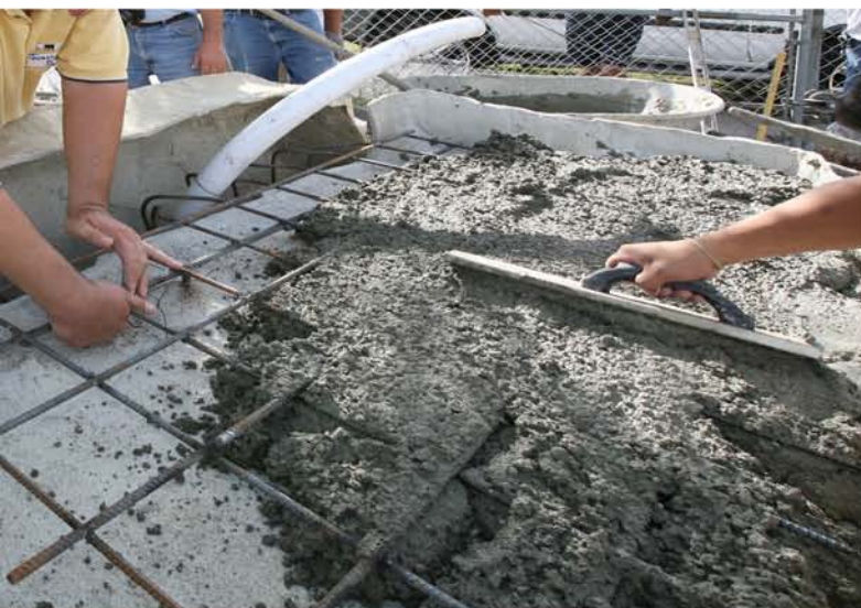
Fill back wall and top with concrete mix, 2000 psi or better. Top should be level. Requires about 1/2 yard of concrete mix.
