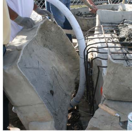
Extend 2 inch pvc plumbing before setting back casting #5. Also run sleeves for lighting.
