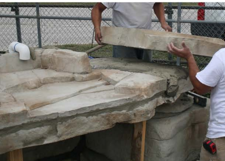
Add 2 inches of concrete fill on each side of grotto top and mortar in top rocks #8 and #9. Add two 90's to 2inch return line to discharge onto grotto top. Set cap rock #10 to hide pipe.
