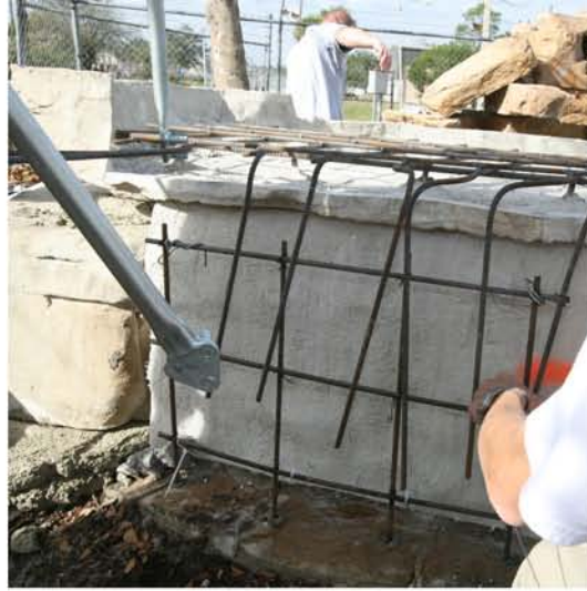
Splice rebar from grotto piece into rebar schedule from pool beam or footing.
