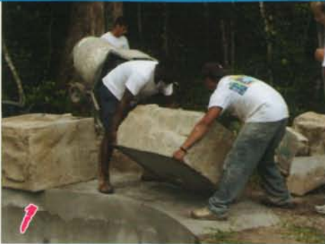
1 Concrete pad should be 12 ft wide, 30" front to back. Dry set base pieces for alignment.
