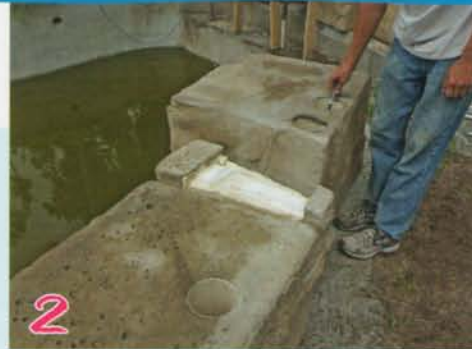
2 Mark concrete pad for rebar dowels. Note "wedge" piece is reversible for radius applications.
