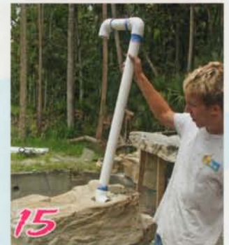
15 Drop in pvc pipe in "pipe" column. Note threaded cap to allow pressure test.
