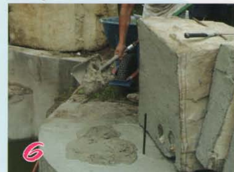
6 One inch mortar bed for base pieces rich mortar, not too wet or too dry.
