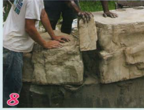
8 Fill gaps between base pieces with small rocks provided with kit for outside radius applications.
