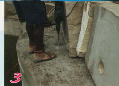
3 Drill holes for rebar dowels. Bond wire needed for steel or use fiberglass rod.
