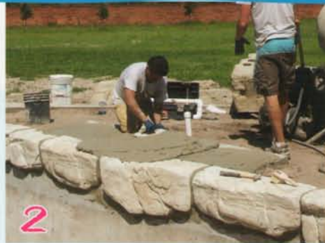
2 Drill and epoxy rebar dowel to concrete pad (center of concrete column) and apply 1" or mortar.
