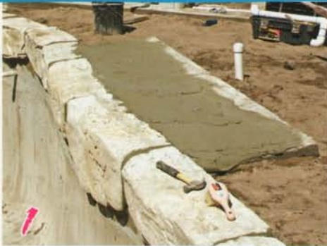
1 Waterfall pad for 3 ft modular should be 7 feet wide, 30" front to back.
